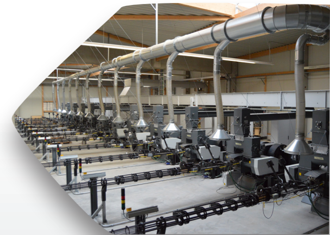
Installation of Holzindustrie Torgau, Germany
