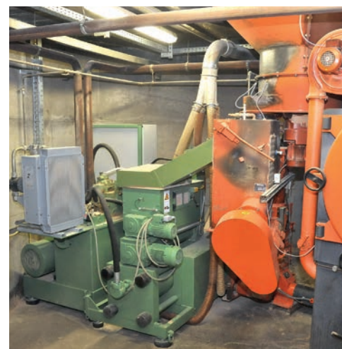
A compact system: The RUF press (left) is installed in a cellar room next to the woodchip boiler.
